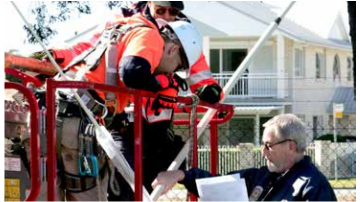
VMRBI Radio Officer John Bodycombe going over the plan for the new radio aerials with the technicians doing the installation.
