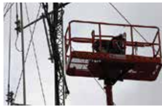
Recently we had a cherry picker on site with the techs from Teleco doing repair work to the tower after the big storm a few months ago and installing another antenna for the upgrade to the radio room.
